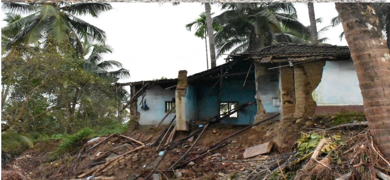
Houses devastated after the flood
